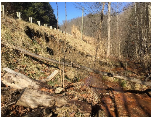
Figure 10: Embankment Failure on Terminal Road
